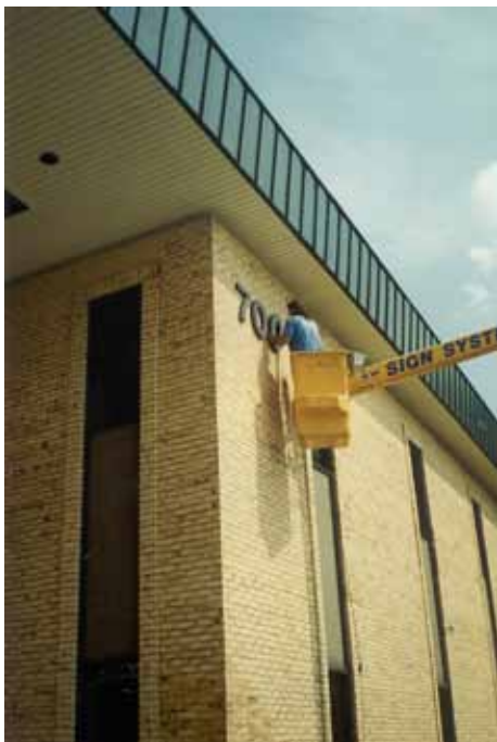
SIGN OF CHANGE: An employee with Sign Systems, Inc. adds the street numbers to the front of NRVCS' Montgomery Center in Blacksburg, as the agency relocated its main operations to that building in the late 1990's. (File Photo)
